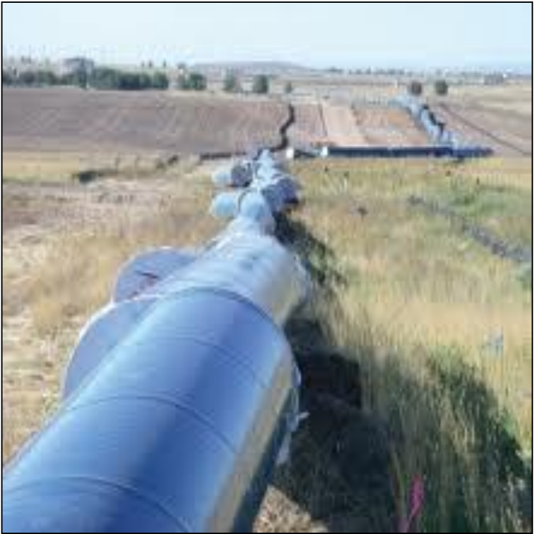
Aurora's "Prairie Waters" Project along E-470
